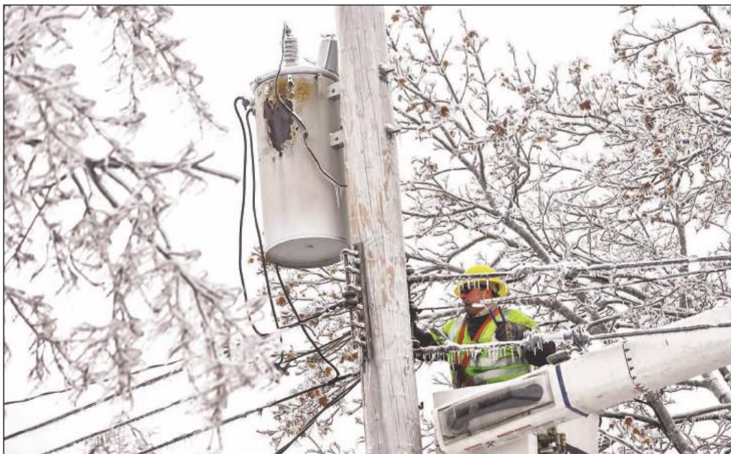
Dave Dora, a lineman from Grand Haven Board of Light and Power, works on connecting fallen wires Monday morning in Lansing. GREG DERUITER/LANSING STATE JOURNAL
