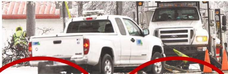
Utility workers are hard at work last week trying to restore power to thousands in the Lansing area. ROBERT KILLIP/LANSING STATE JOURNAL
