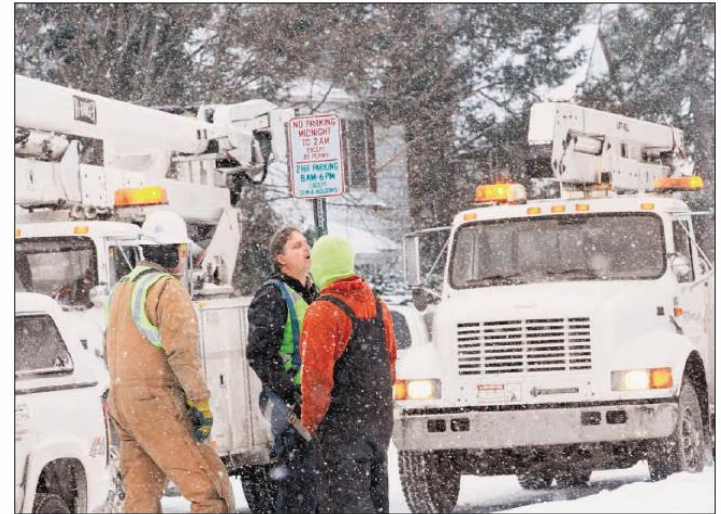
Crews from Fox Power of Gladstone in the Upper Peninsula respond to a service call Wednesday at a home in East Lansing. The crews were helping out Lansing Board of Water & Light customers with problems caused by the ice storm. GREG DEWITT/LSJ
